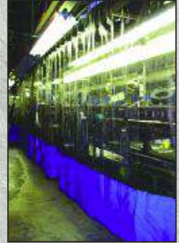
Tire Processing Containment System
