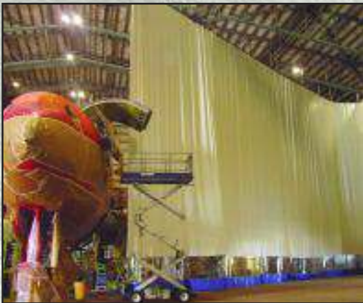
Aircraft Overhaul/Finishing Spray Areas
